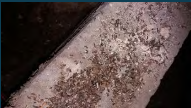
Extensive bat droppings under the ridge board
