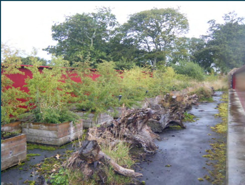
Planters and tree stumps on bridge deck
